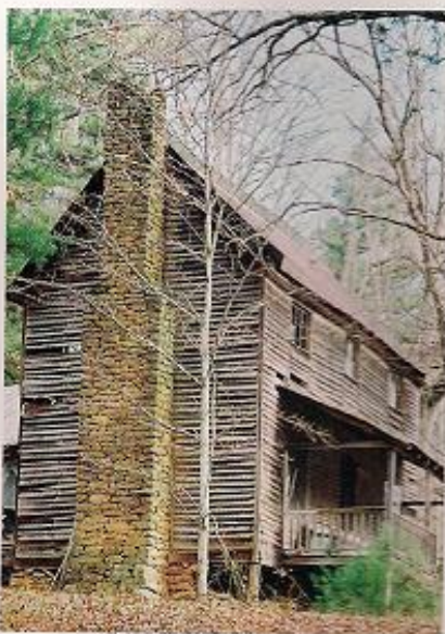
The abandoned home built by David Pace at Camp Creek, the original settlement of what became Saluda.
